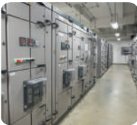
Electrical Control Panels
